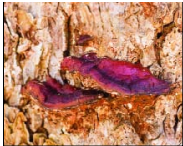
Conks of decay fungus indicate a loss in wood strength.
